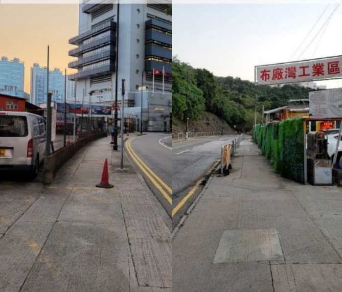
Widening and facelifting of footpaths along western side of Shum Wan Road 擴闊及美化深灣道西邊行人路
