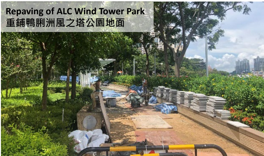
Provision of new seating at ALC Wind Tower Park 於鴨脷洲風之塔公園提供新座椅
