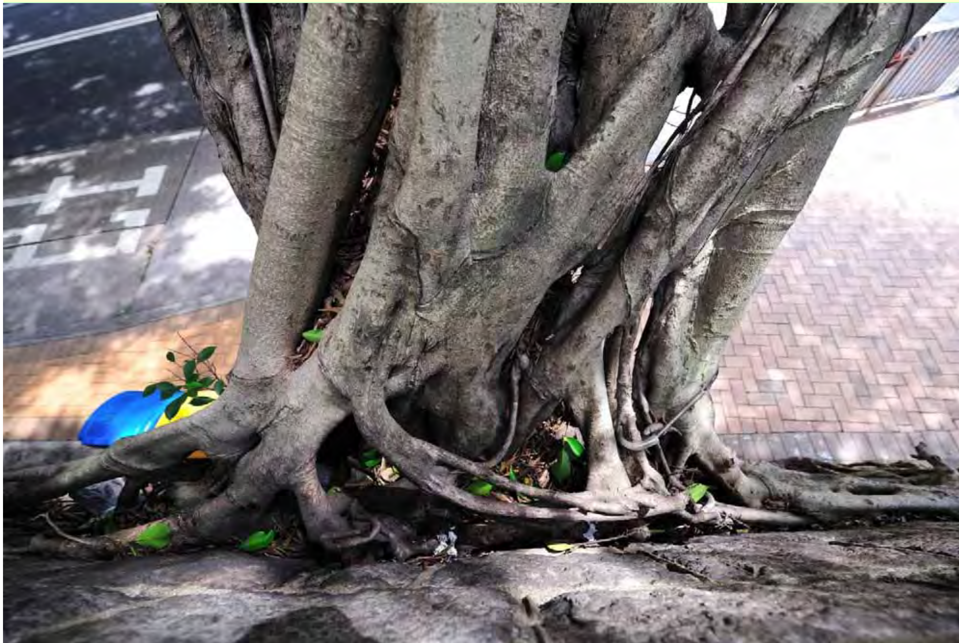
Photo T6-7. Relationship between tree and wall crest, viewed from the south.
