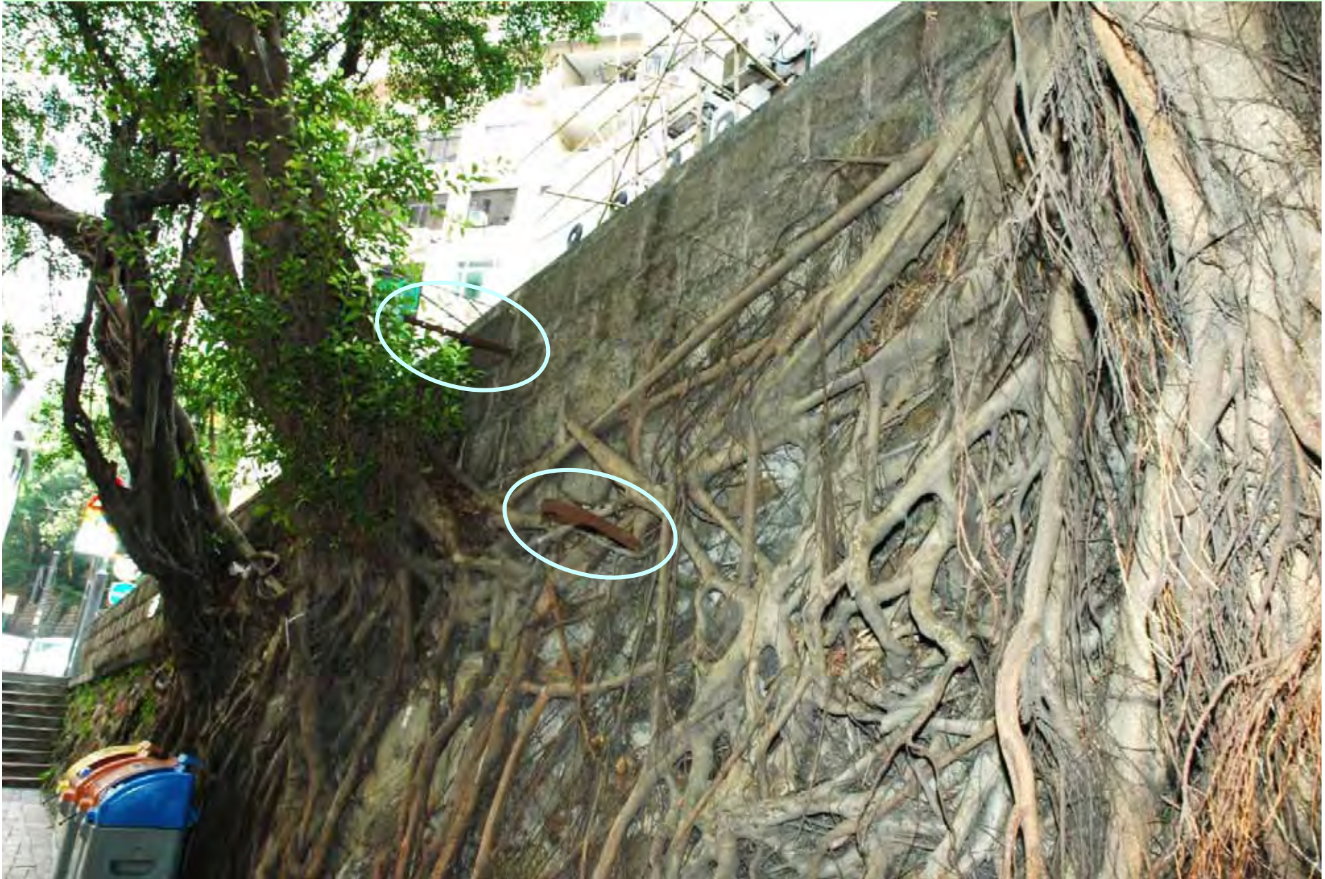
Photo T4-13. East side of surface root mass with obsolete angled iron installation.
