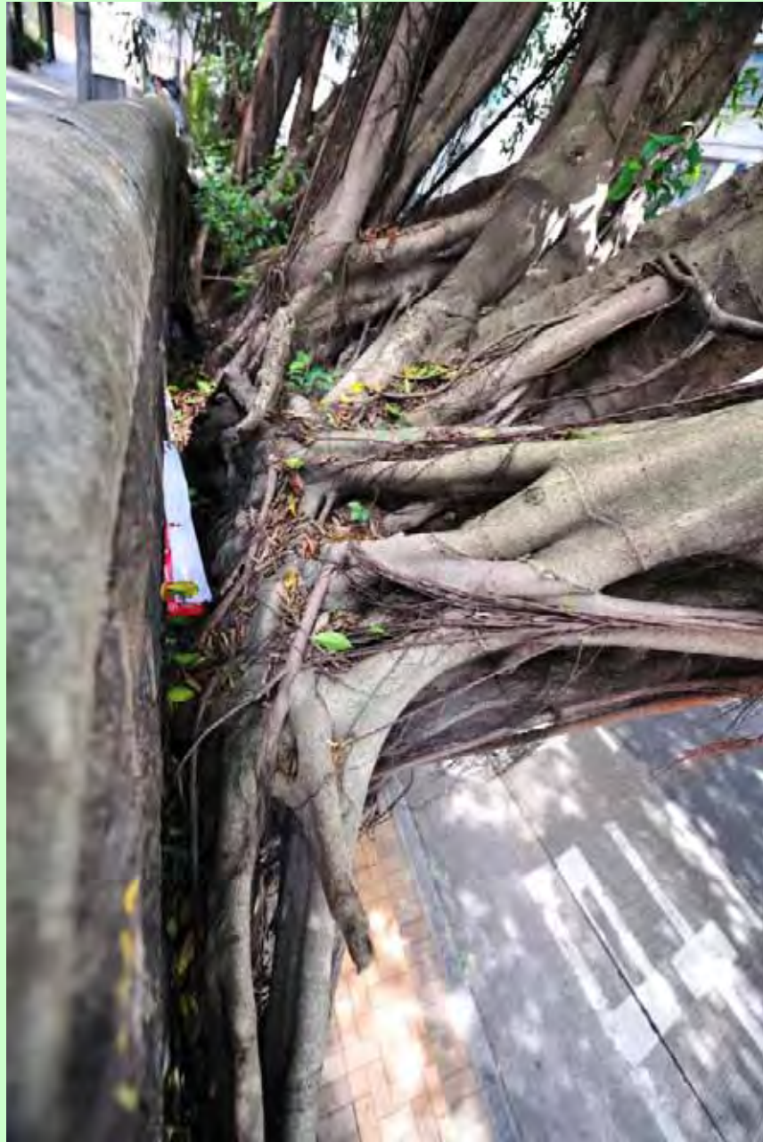
Photo T4-11. Partial detachment of tree based from wall crest, close-up view from the east.
