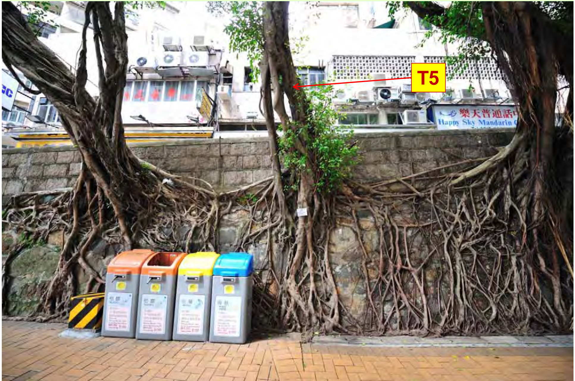
Photo T5-4. Limited spread of surface roots and their grafting with neighbours T4 & T6, and restriction to root penetration at wall toe.
