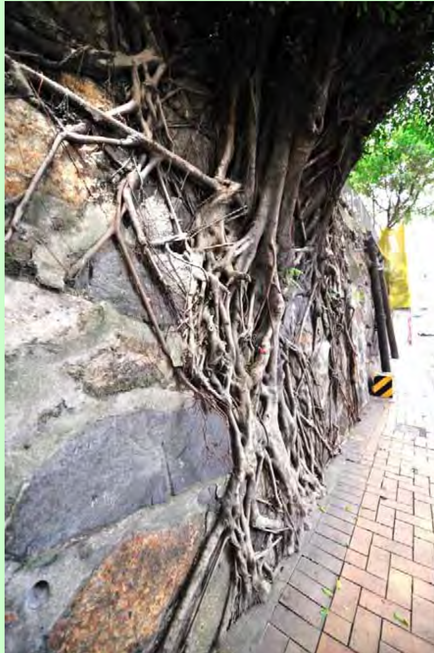
Photo T2-11. Restriction to root penetration at wall toe.
