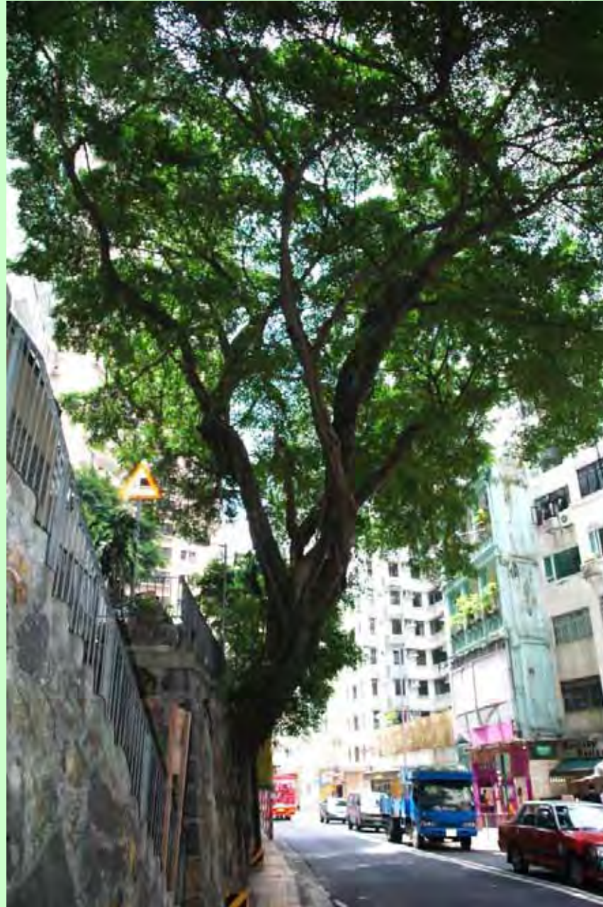
Photo T2-3. The large upright tree anchors at the crest of the west side of the old stone wall, hanging above the carriageway.
