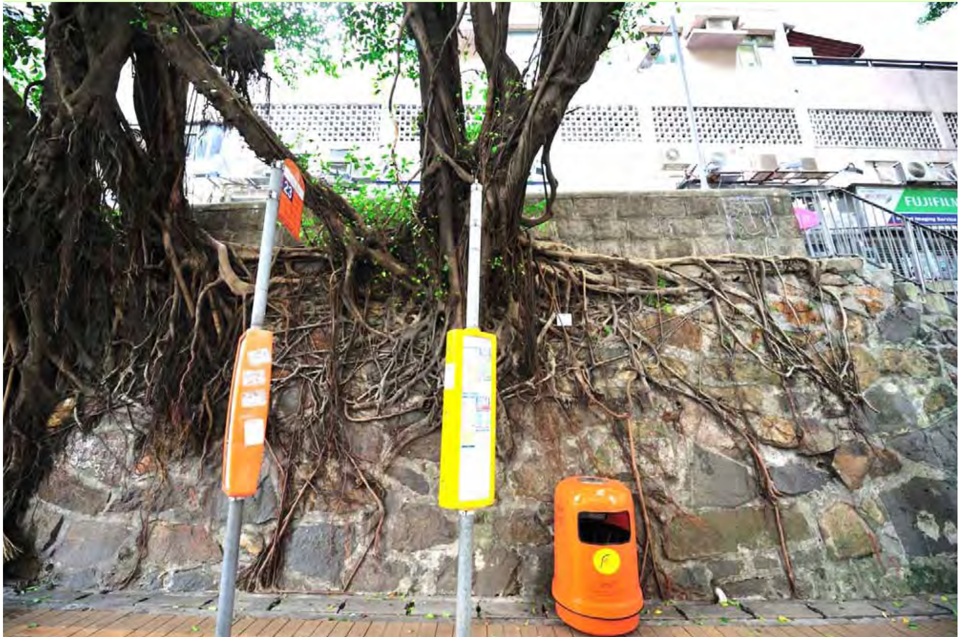
Photo T3-7. Limited spread of surface roots, cement filling of wall joints, and restriction to root penetration at wall toe.
