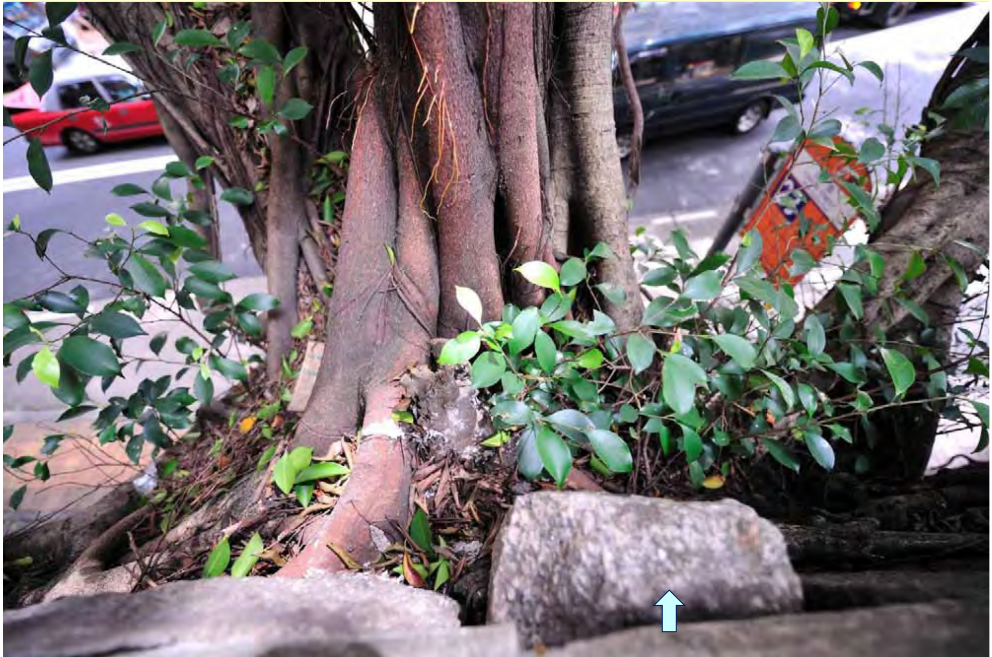
Photo T3-10. Relationship between tree and wall crest, viewed from the south. Shifted masonry block.
