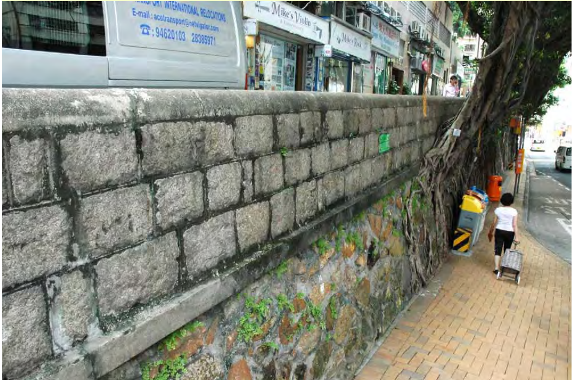
Photo T6-6. Restriction to root penetration at the toe of the rather low retaining wall.
