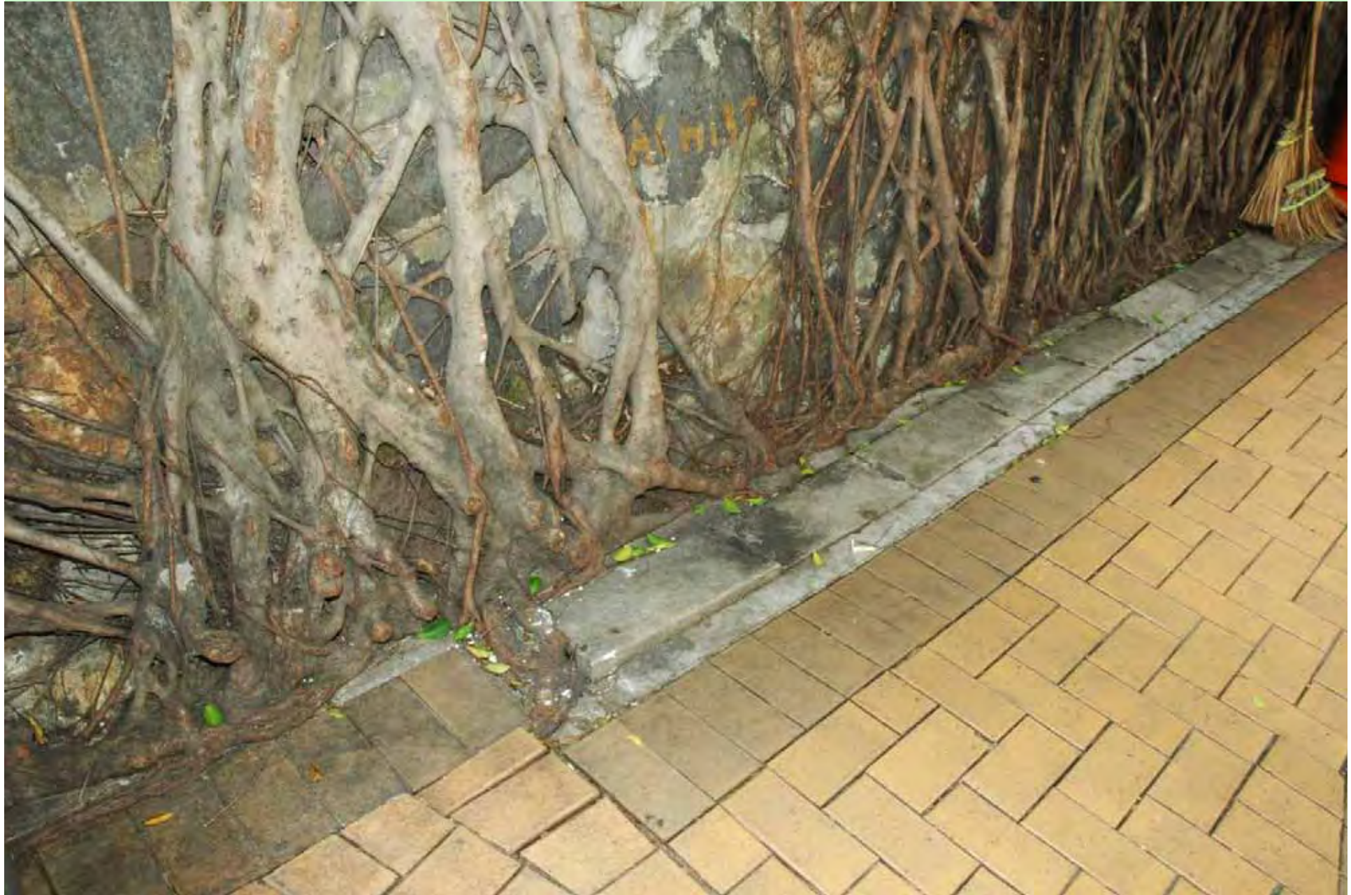
Photo T4-7. The drainage channel at the wall toe restricts root penetration into the soil below the pavement.
