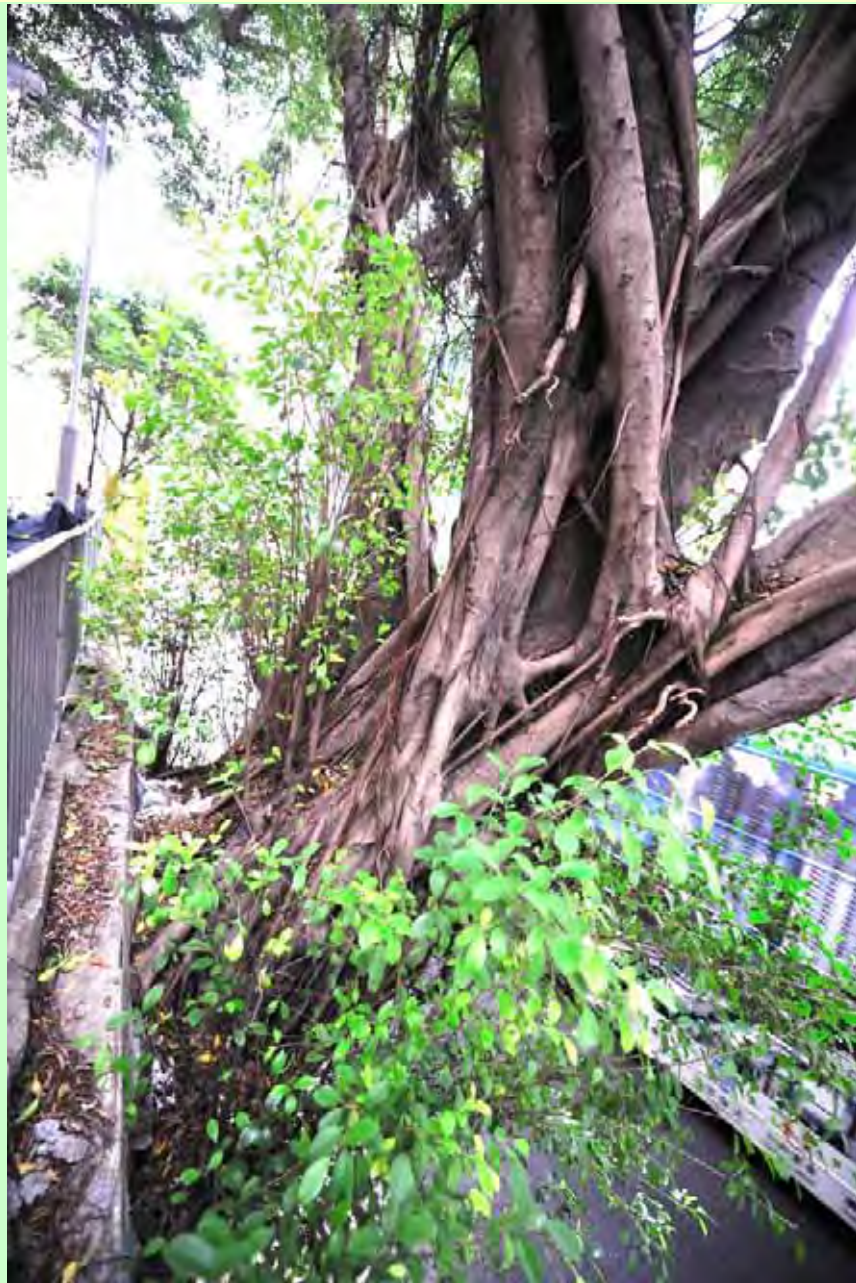
Photo T2-12. Relationship between tree and wall crest, viewed from the east.
