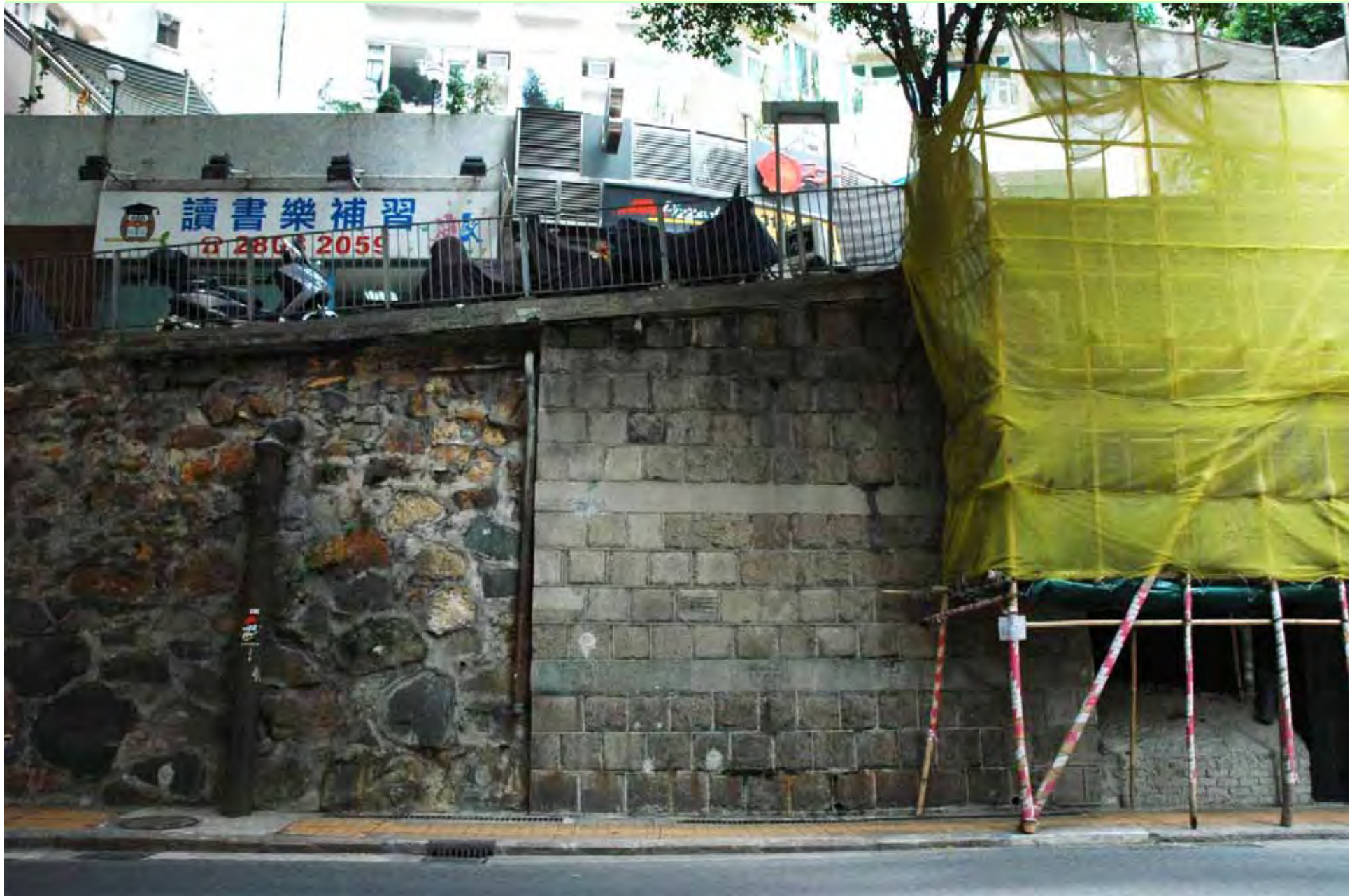
Photo T1-4. The wall section has regular squared-dressed granite blocks, contrasting with volcanic rubble boulders of the main wall.
