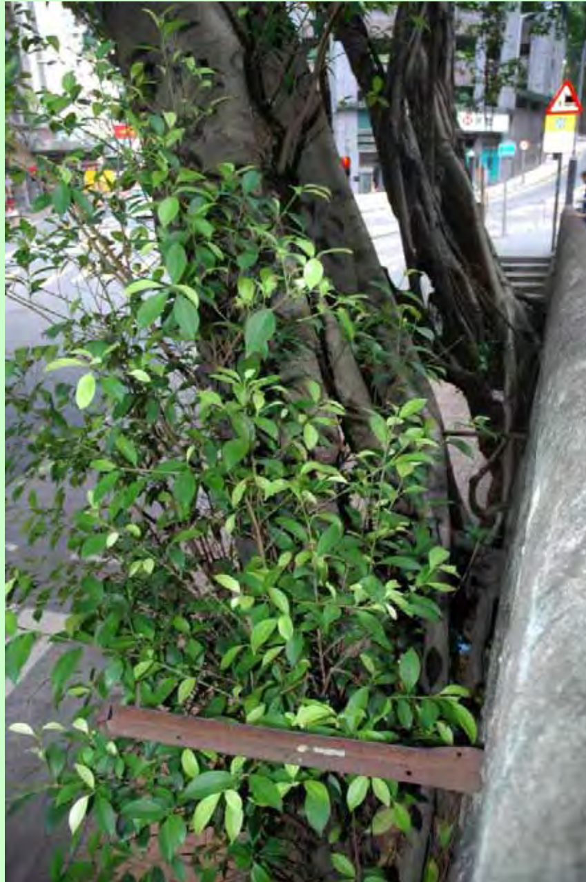
Photo T5-6. Relationship between tree and wall crest, viewed from the west.
