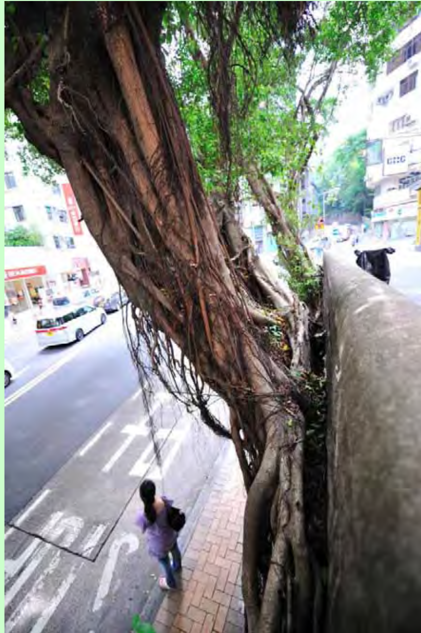
Photo T4-8. Partial detachment of tree based from wall crest viewed from the west.
