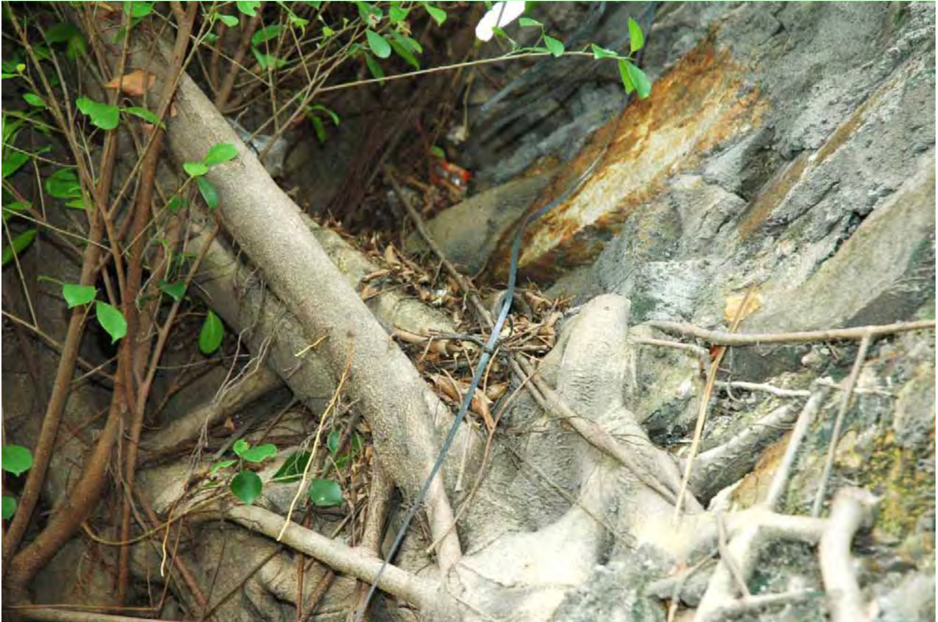
Photo T2-18. West side of the surface root spread near the trunk base indicating slightly protruding masonry blocks.
