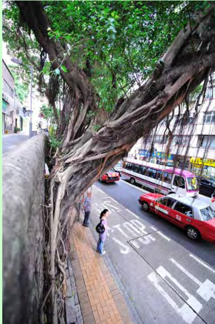
Photo T4-9. Partial detachment of tree based from wall crest viewed from the east.
