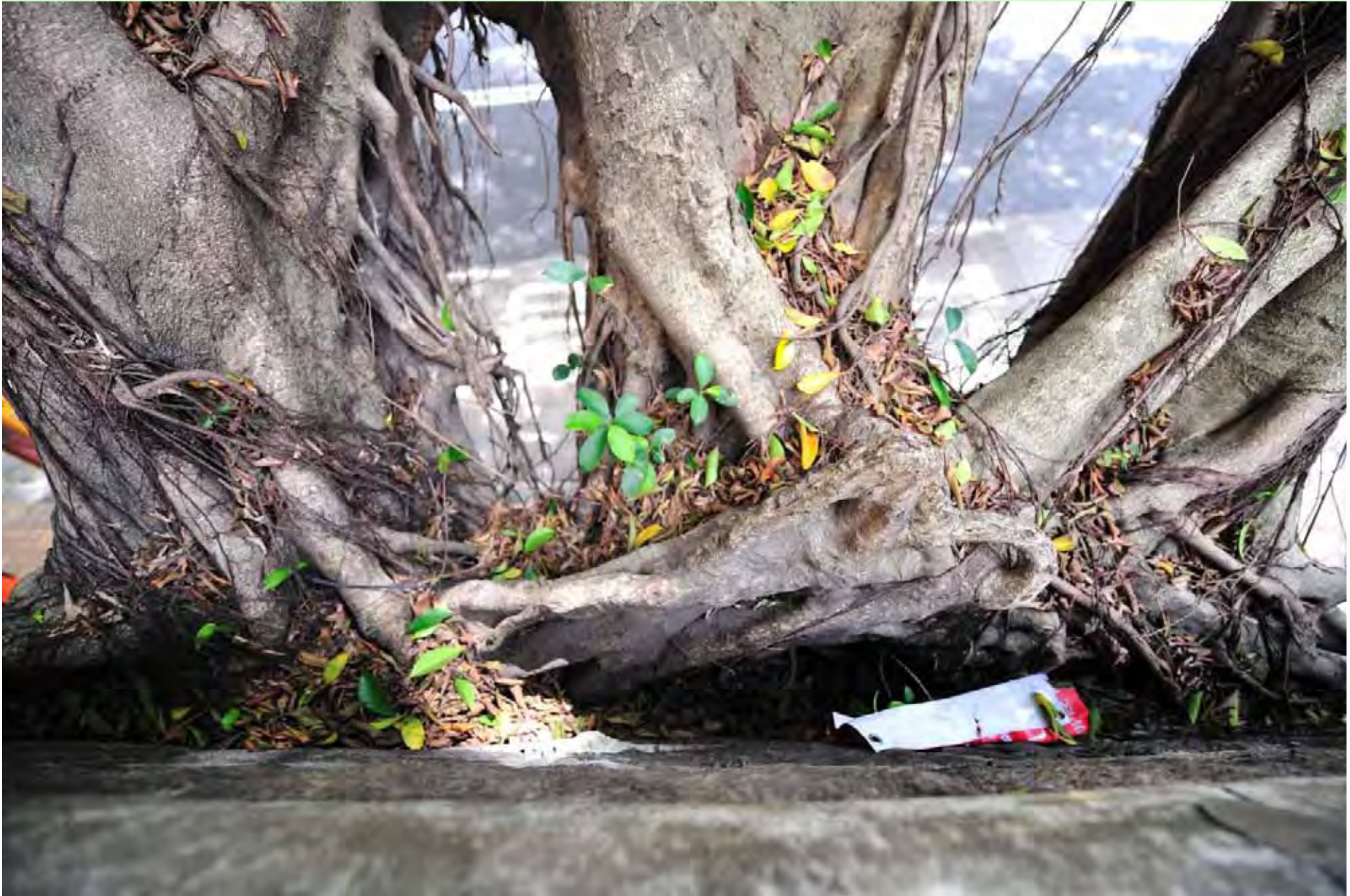
Photo T4-12. Partial detachment of tree based from wall crest, close-up view from the south.
