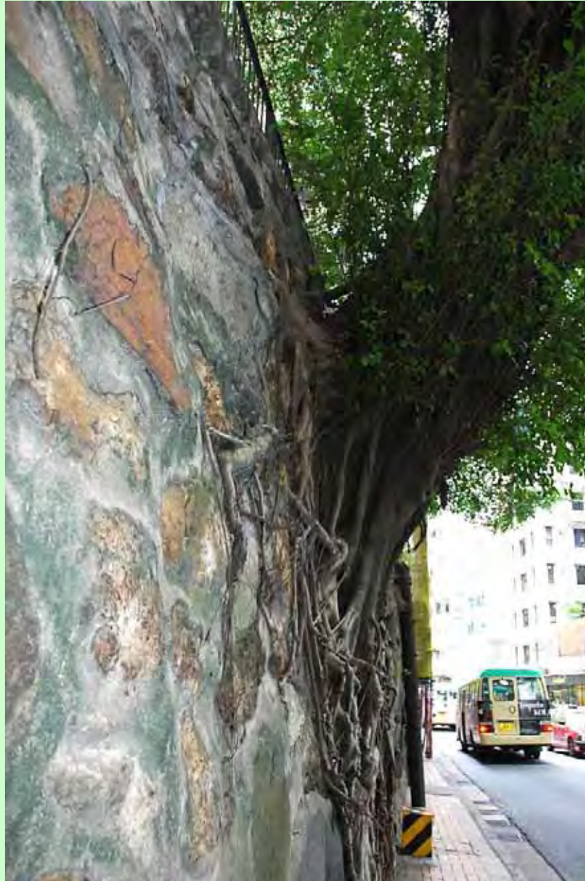
Photo T2-15. East side of surface root spread indicating slightly bulging surface of masonry blocks and cement sealing of joints.
