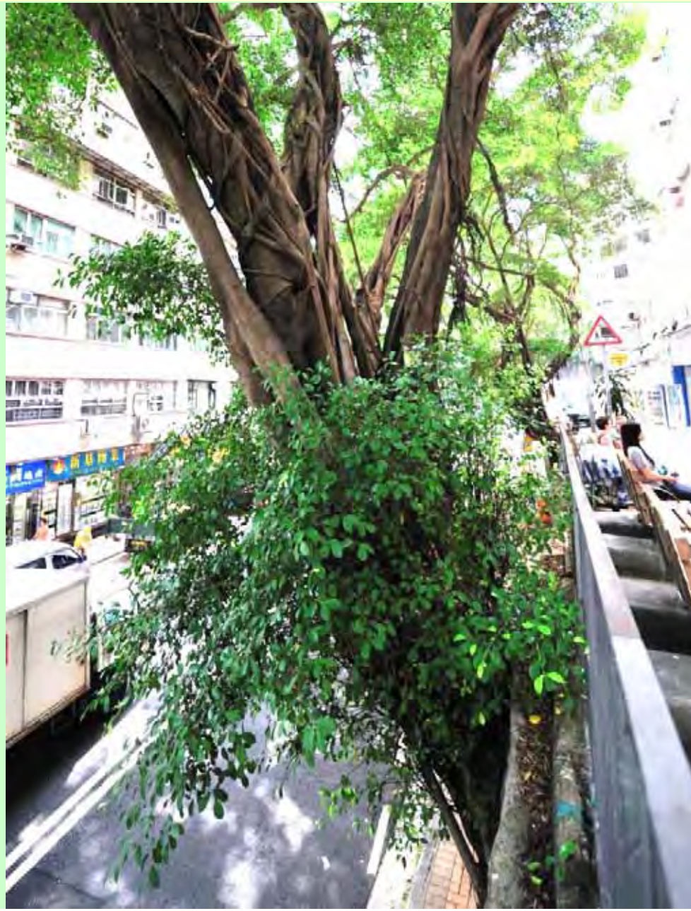
Photo T2-13. Relationship between tree and wall crest, viewed from the west.
