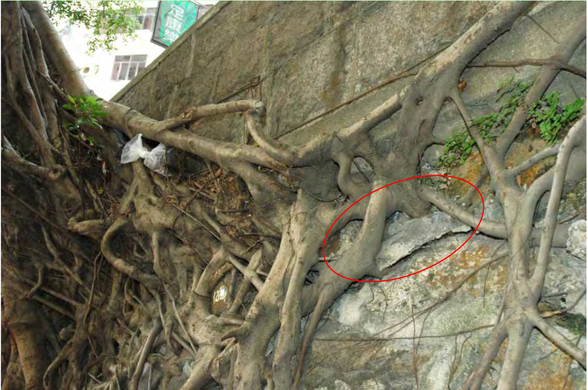
Photo T6-9. Surface root mass on the west side with loosened mortar. Litter accumulation in surface roots.
