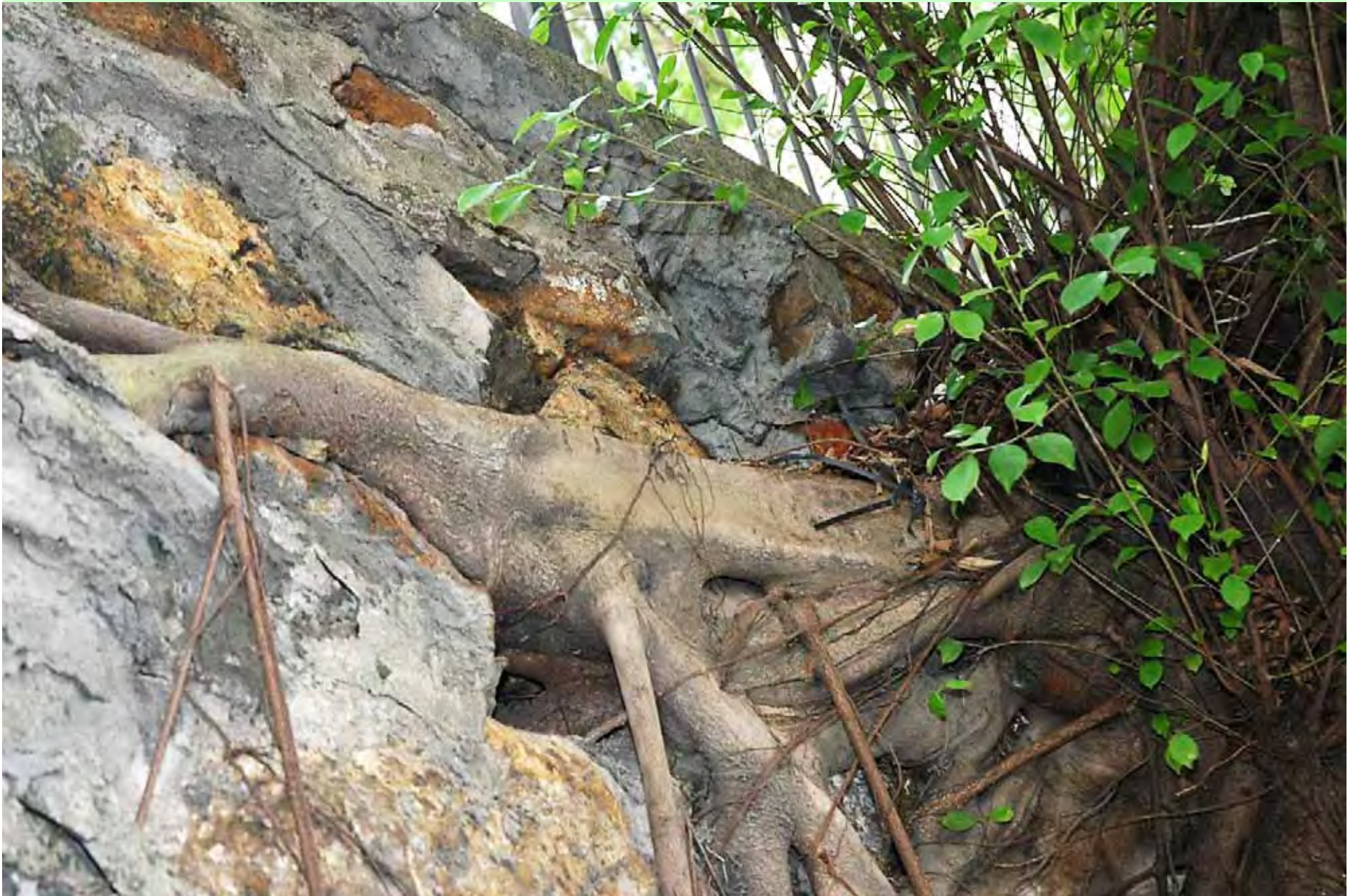
Photo T2-16. East side of the surface root spread near trunk base indicating displacement and omission of masonry blocks.
