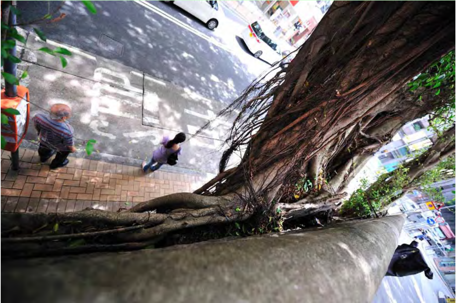
Photo T4-10. Partial detachment of tree based from wall crest, close-up view from the west.
