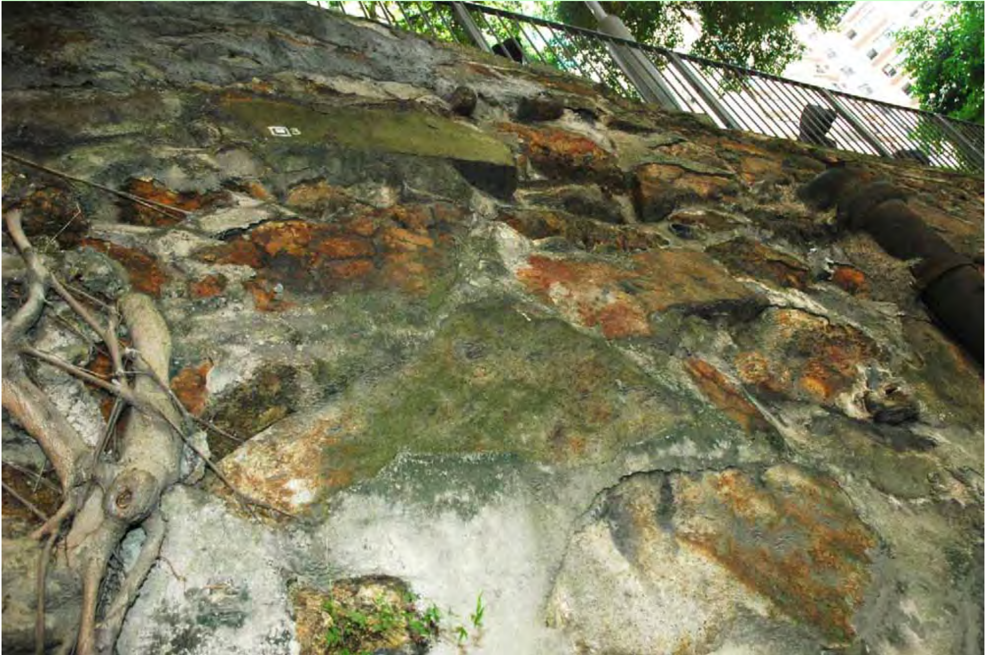
Photo T2-19. West of the surface roots showing uneven surface and new cement pointing of the rubble wall.
