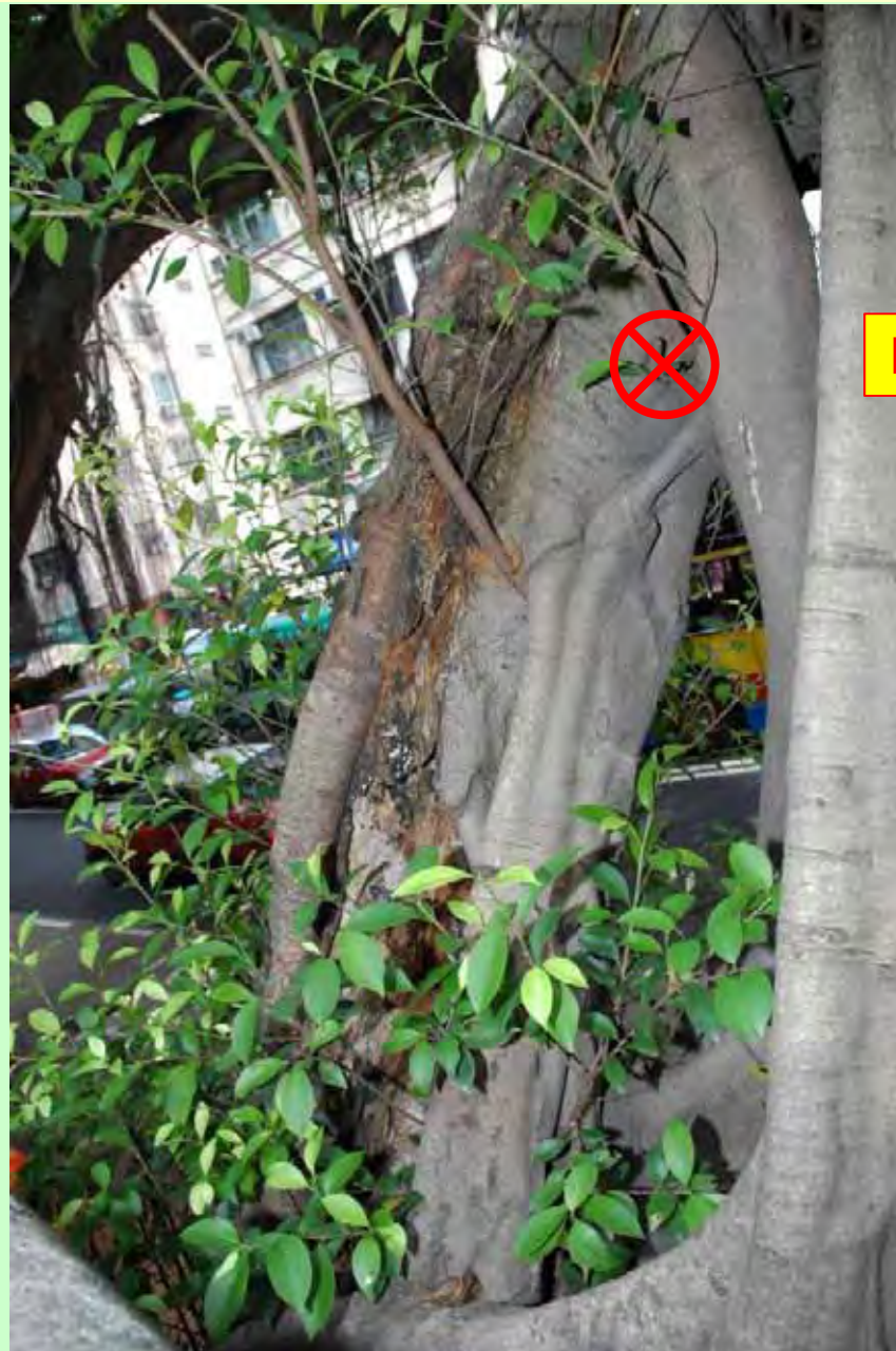
Photo T5-9. Upper end of the trunk cavity with upward extension of wood decay. Cross denotes drilling position.
