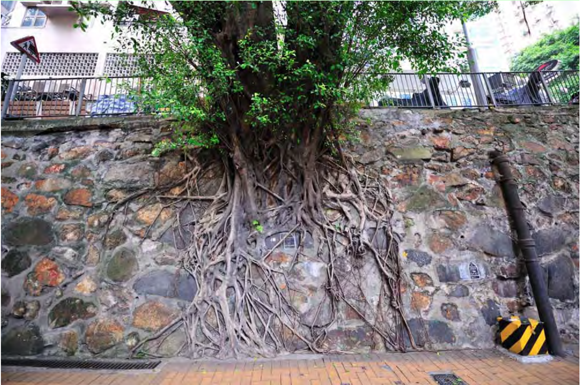
Photo T2-10. Limited spread of surface roots on the stone wall face.
