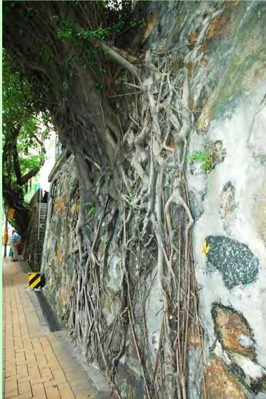
Photo T2-17. West side of the surface root spread indicating extensive buttering of joints by cement.
